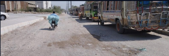
Existing condition — the carriageway on Road 10000, Korangi.
